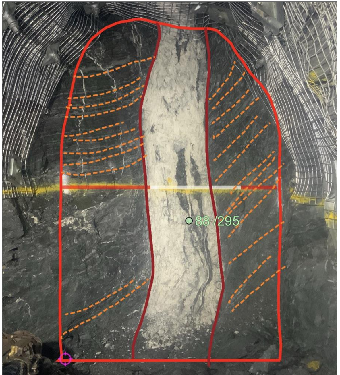
Figure 7.11: A well-developed Shepherd gold-only vein in the 600 lode face, Youle 617 Level at 7014N looking south
